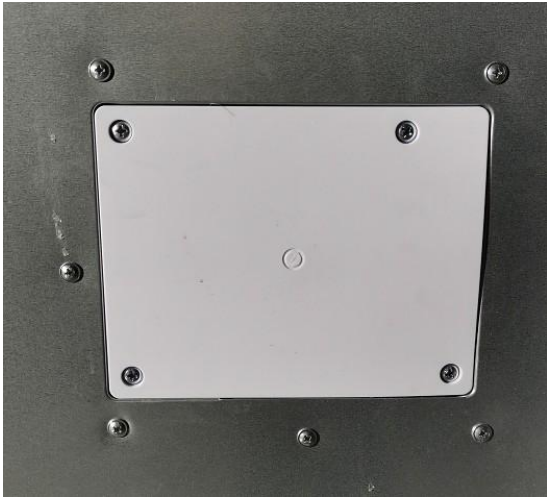
Rear Access Panel
