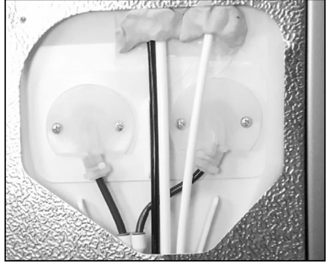
Fill Tube Heaters & Water Lines
