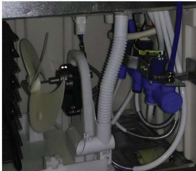
Fridge water drain group
